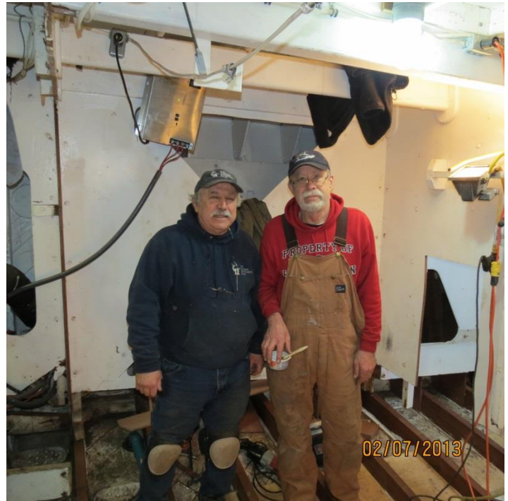
Jim Lyons & Ron Taylor "PT Boat Shipwrights" standing on new shaft log and frames in aft tank room
