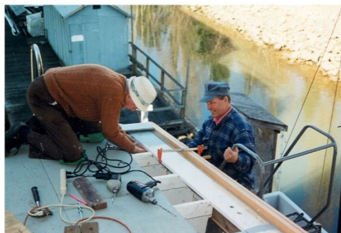
Bob Hostetter and Ron Reichardt begin fastening two layers of 2" by 6" Douglas-fir planks to provide gunwale rub rails the full length of the boat on both sides.
